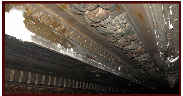
The plasterwork in May 2010, pre-restoration.
