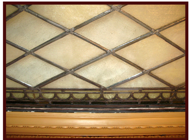
Restored and repaired panes of glass. Note the hint of yellow in the border—it is repeated in the centerpiece of the skylight.
