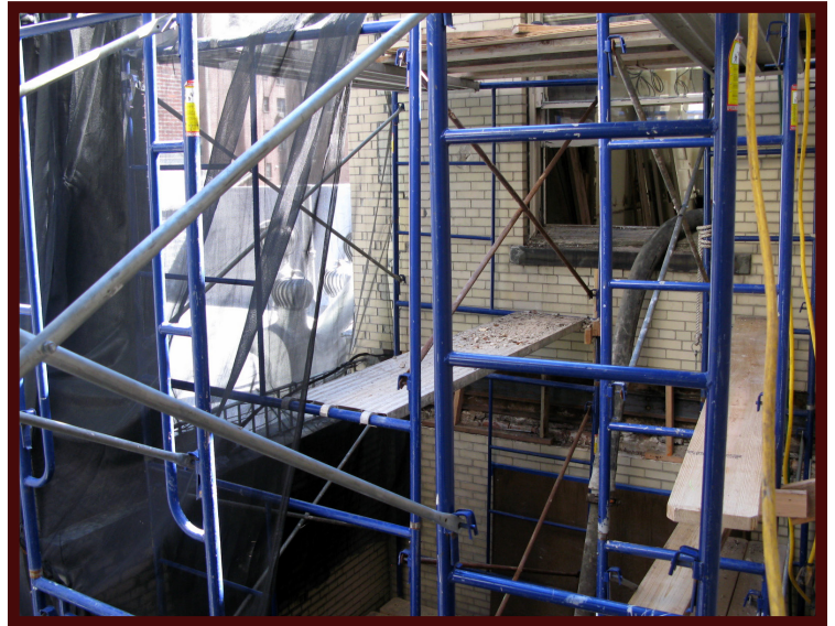
Look closely and you can see a hose coming through the window and down the side of the building.
