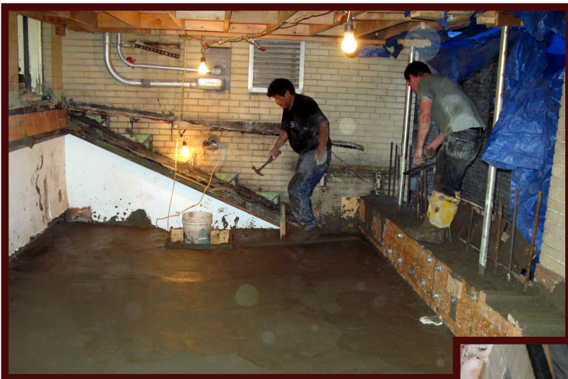
30M Construction president John McBride (right) and a workman after the first concrete pour.
