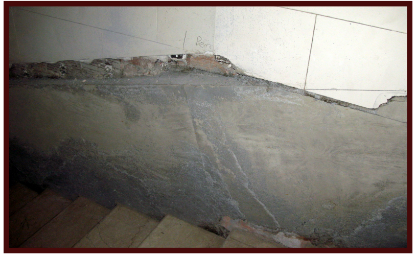
Above: The west wall fully reinforced and ready to bear the weight of the Handi-Lift.
