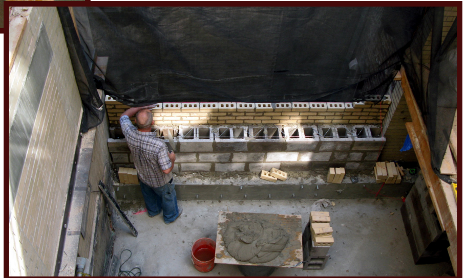
One of the workmen bricking up the new east wall of the building.
